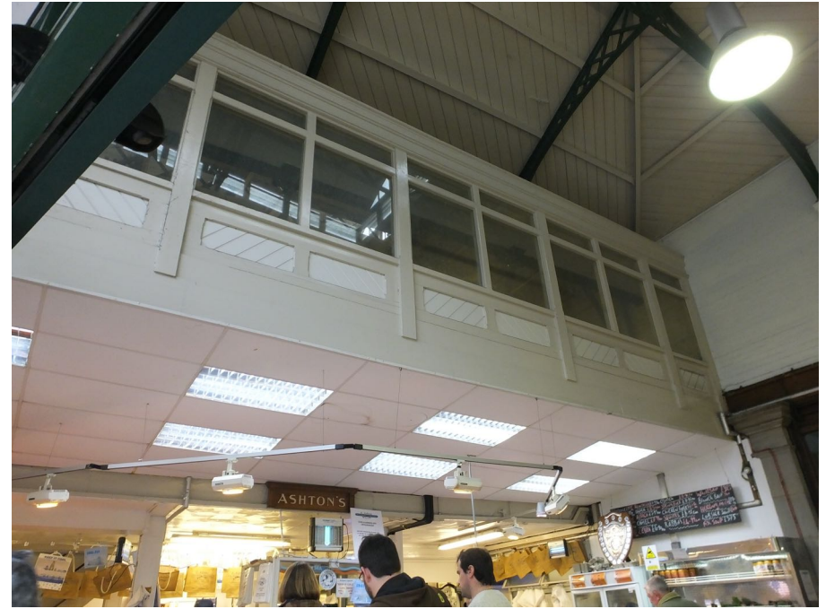
View of the added mezzanine first floor structure and screen which is to be removed. Note the visible elements of the finely detailed roof structure of the original fish market above.
